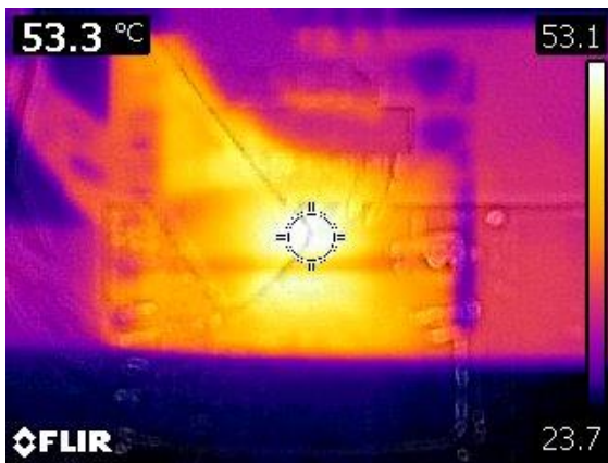
Fig. 10. Measuring the temperature of the inverter by thermal imaging
