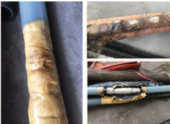
Fig. 3. Disassemble and inspection of the fault cable
